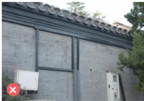
管线线槽过于突兀
